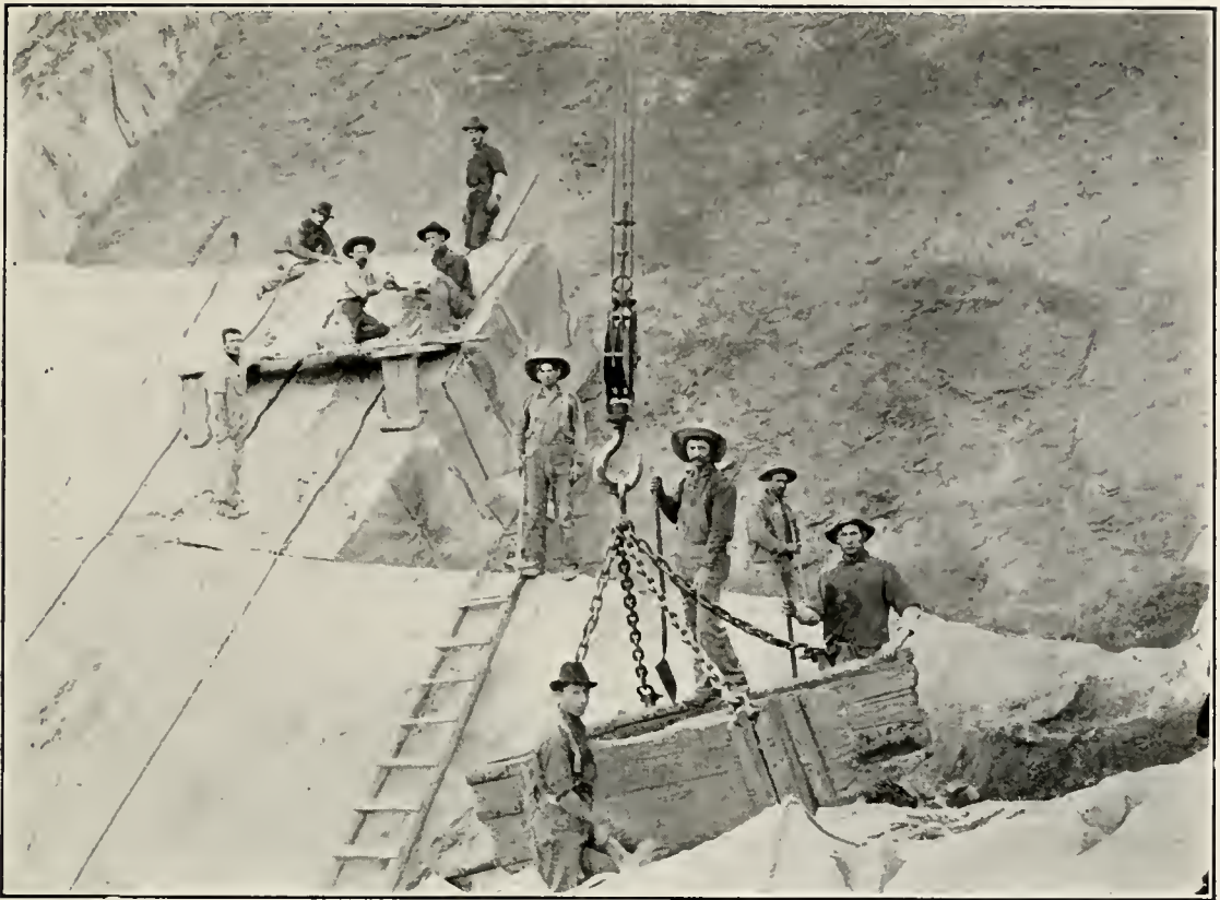
ILL. No. 54. A PORTION OF THE FACE OF THE MCGILVRAV SANDSTONE QUARRY, COLUSA COUNTY.
