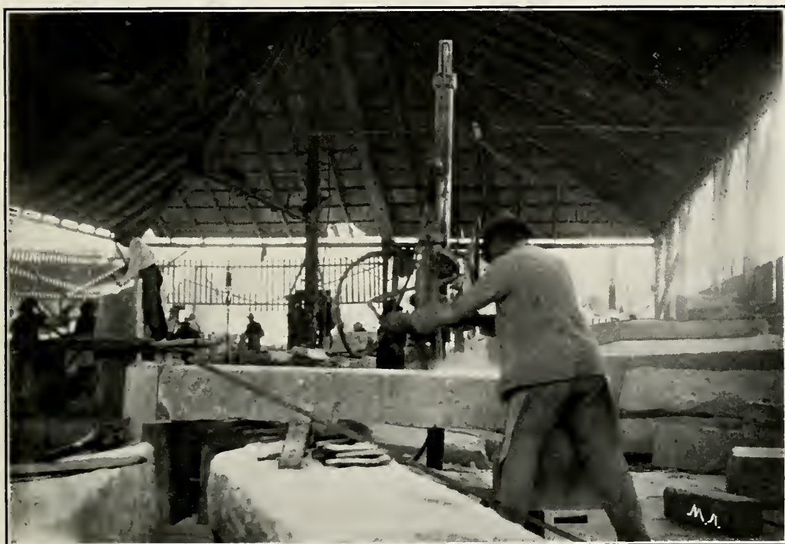
ILL. No. 13. MACHINE SURFACING GRANITE AT BLY BROS.' STONE YARDS, LOS ANGELES.
