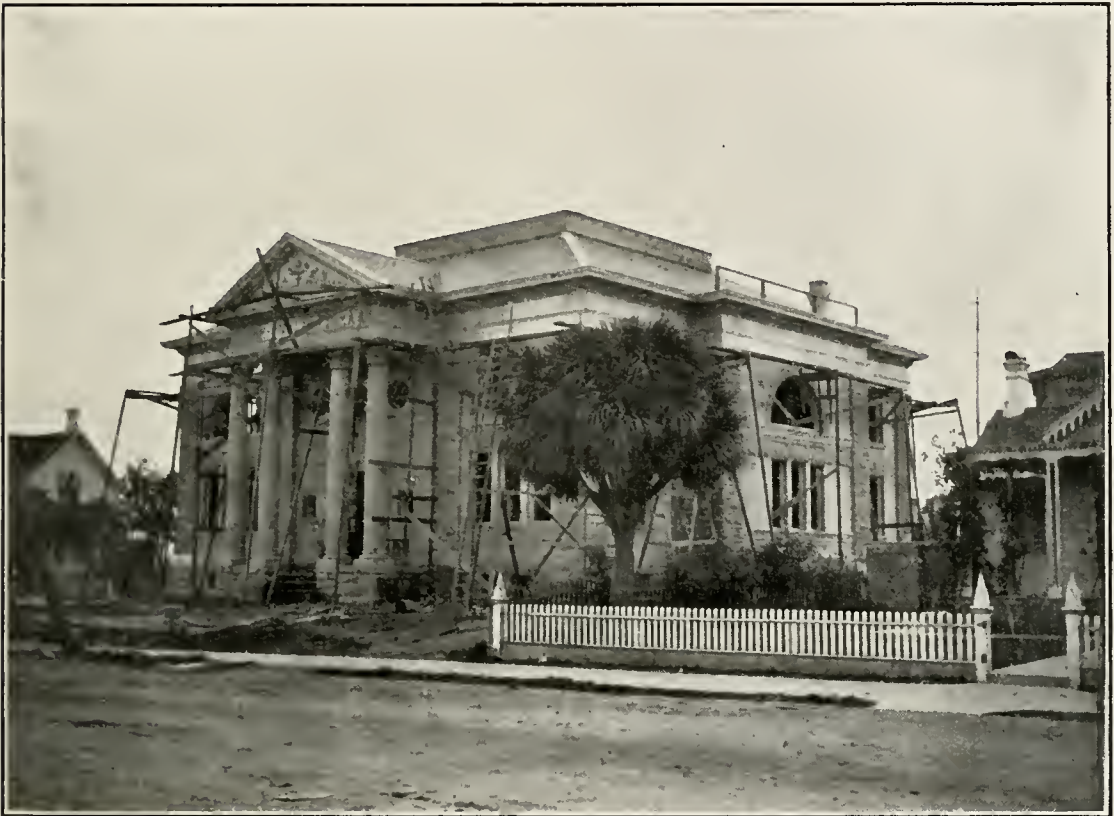
ILL. No. 76. CARNEGIE LIBRARY, PETALUMA. Constructed of Trachytic Tuff from Stony Point Quarry.
