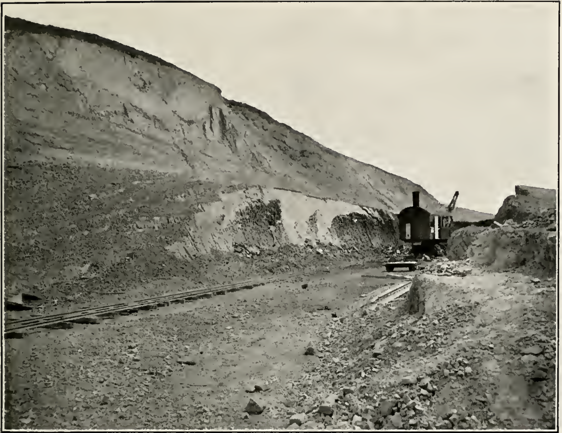
ILL. No. 84. STEAM SHOVEL AT WORK IN CLAY PIT, PACIFIC PORTLAND CEMENT COMPANY, CONS., SOLANO COUNTY.
