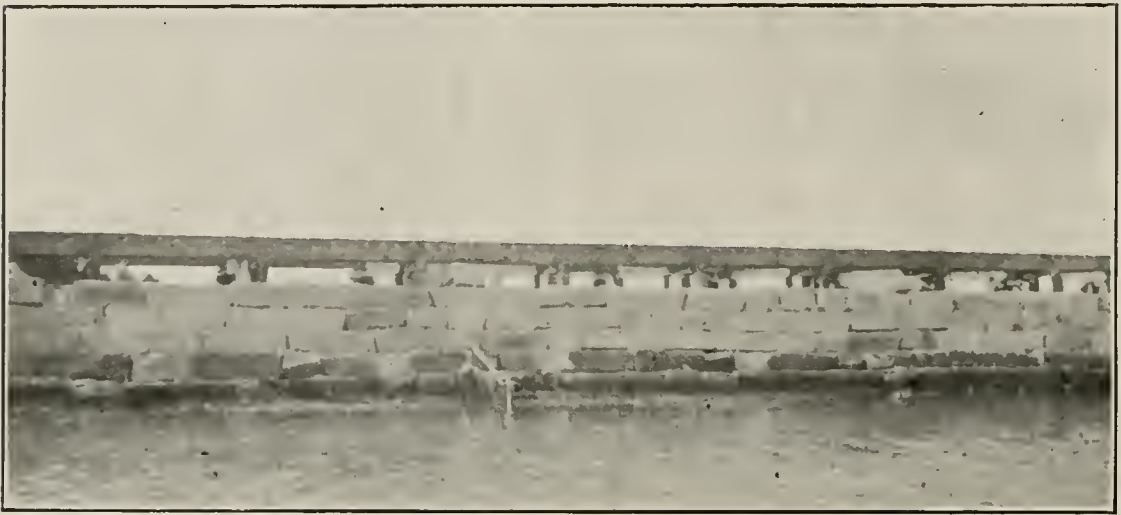
ILL. No. 140. VIEW OF HARBOR SIDE OF SAN PEDRO BREAKWATER. Granite blocks (over 6000 pounds each) from Casa Blanca Quarries, Riverside County.
